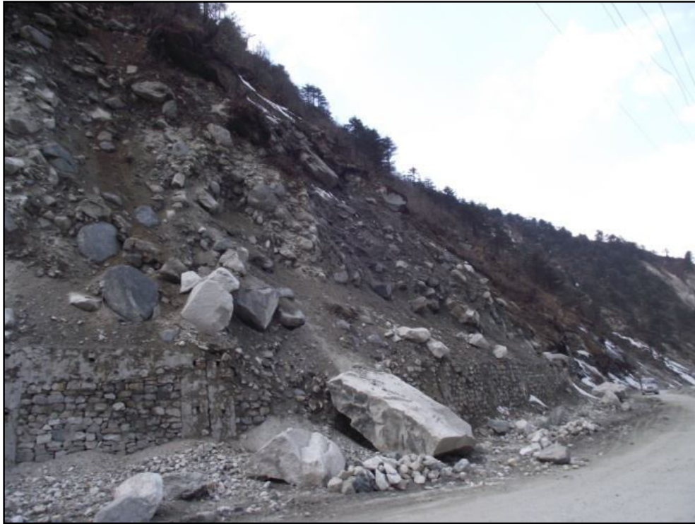
Picture 3 Debris fall triggered by Ground vibration due to Vehicle Movement
