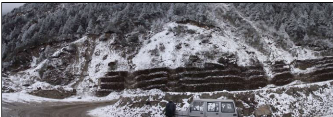
Picture 8 Partial collapse of the Retaining Structure due to Debris slide
